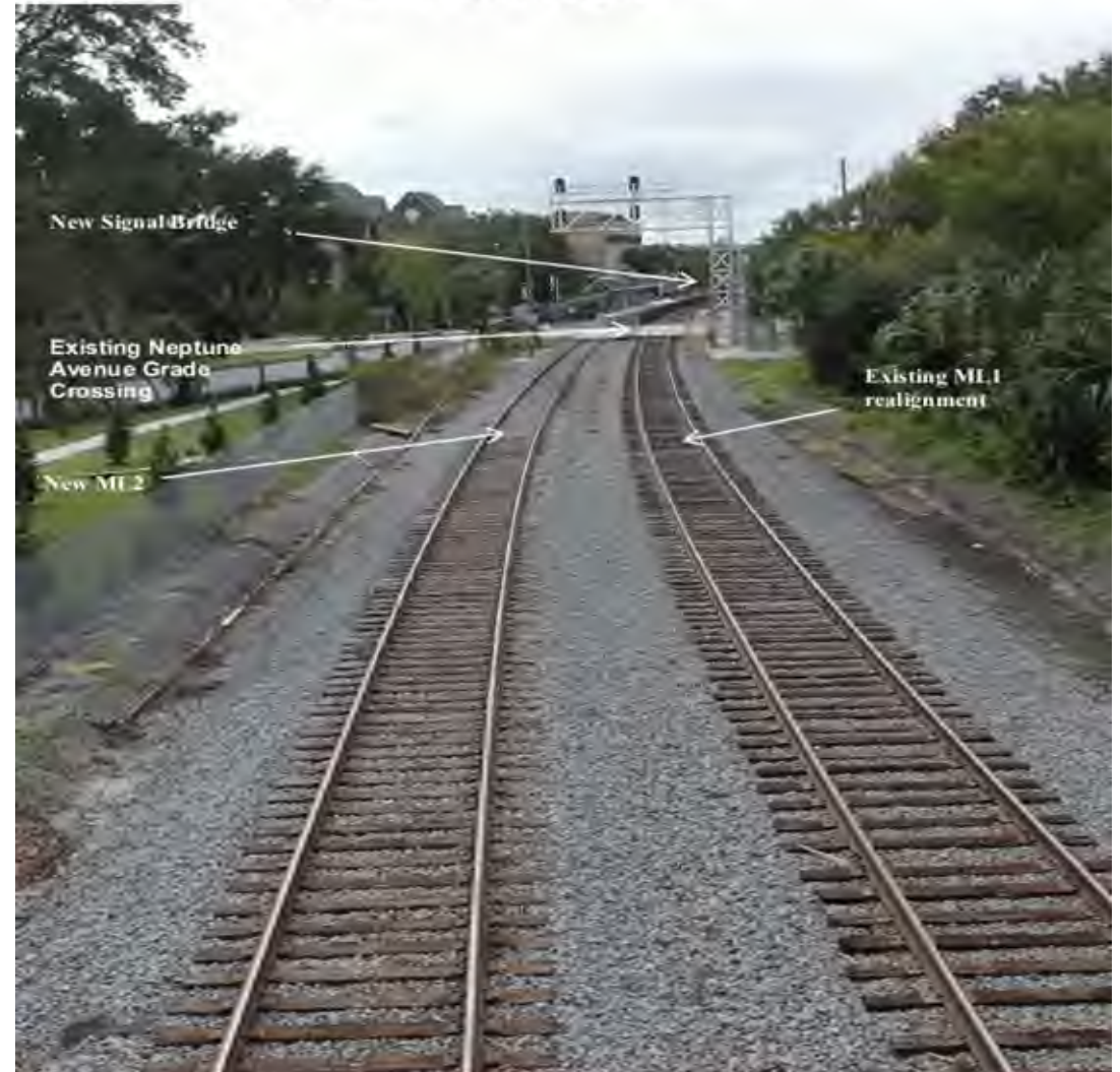
Looking South at Neptune Grade Crossing - End of CRISI P2S Double Track Project
