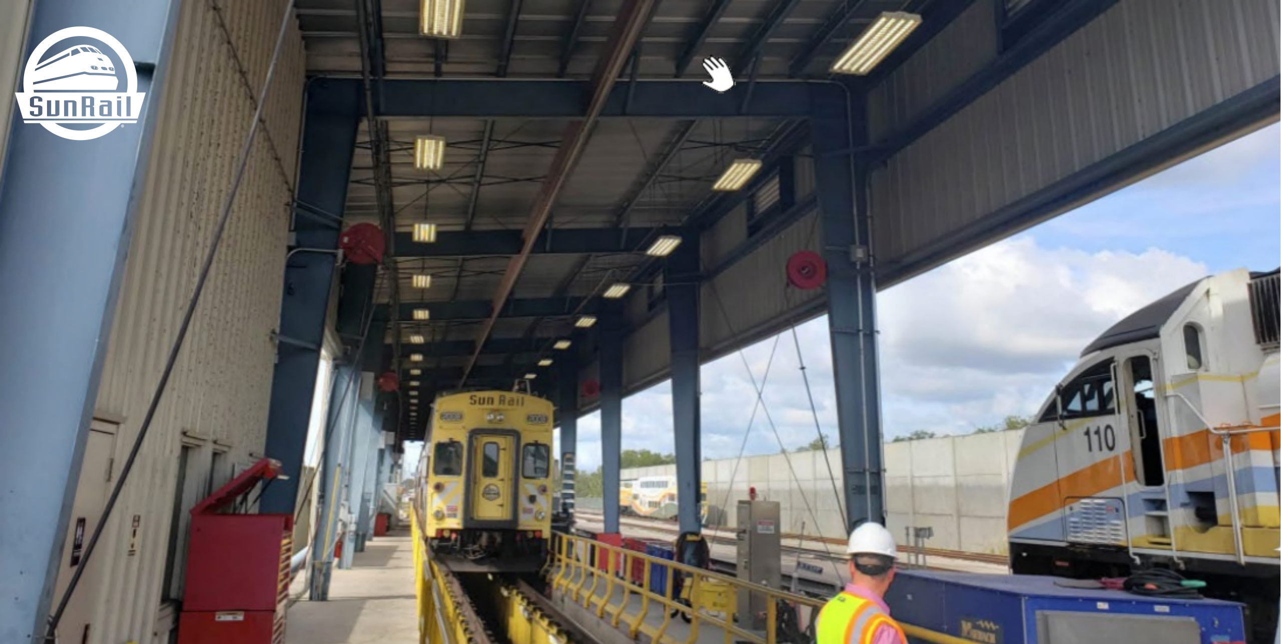
VSMF Service and Inspection Pit
